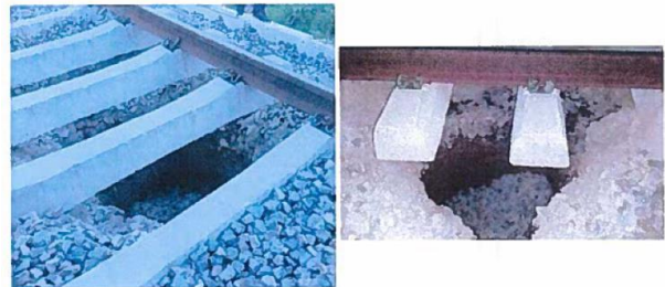
Figure 10 Safety problem on the rail track
